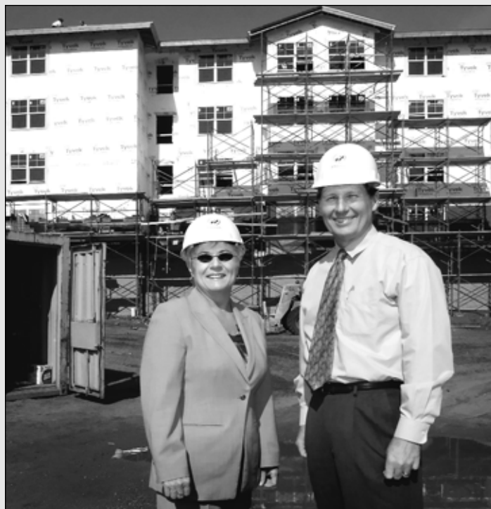
Fran Bly and Marvin Plakut review the progress at Carty Heights . We're on-track to open in the fall with all 49 apartments spoken for.
